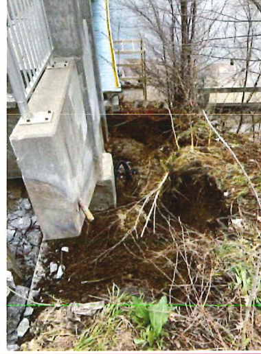
Erosion and undermining around bridge wing and abutment slope
