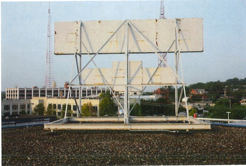
Figure: The view from the rooftop looking southwest at the rear of the sign shows the metal structure.
