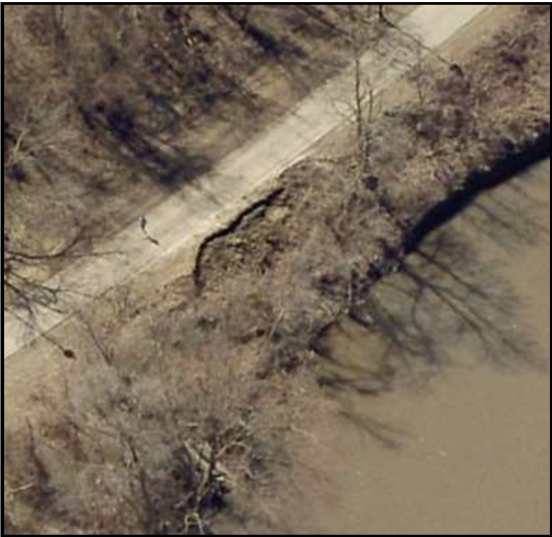
Photo Above: Oblique Aerial of Landslide
