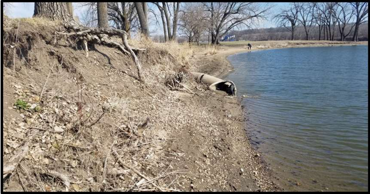
North-centrally located 6-foot tall eroded lake shoreline and damaged storm sewer.
